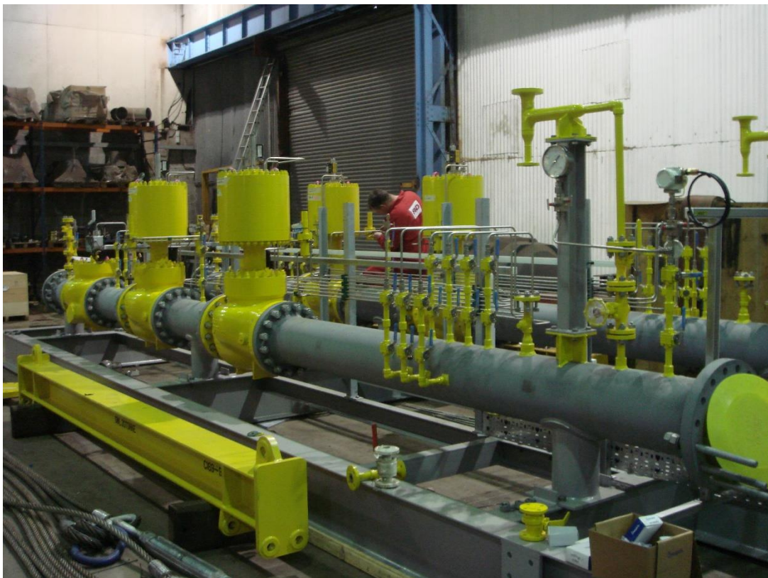
Fig 3.2.1 Installation of control valves series HON R100 in skid mounted pressure control and protection system
